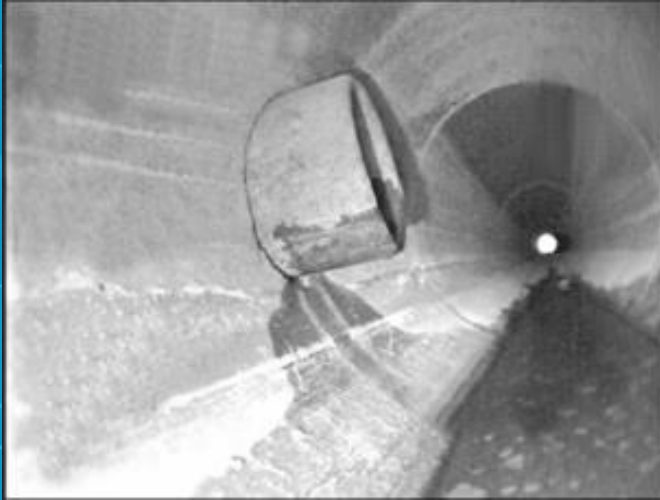
Negative slope obstruction
